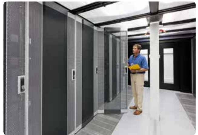
Indirect adiabatic cooling ensures highly efficient cooling to server racks.
