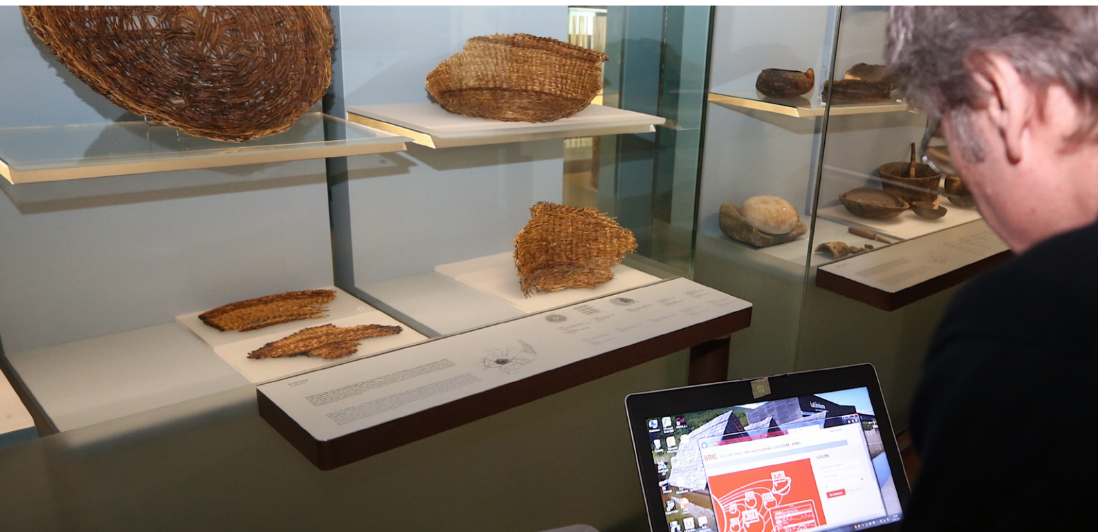
Christian Cevey can connect directly to the climate control software from the permanent exhibition.
