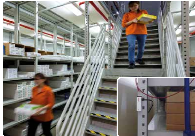
RMS Mini Logger installed in the warehouse.
