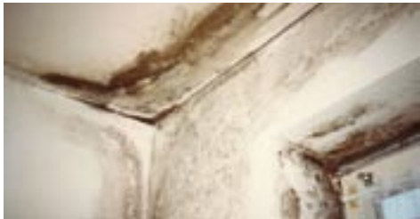
Mould caused by thermal bridges in a flat in an old building
