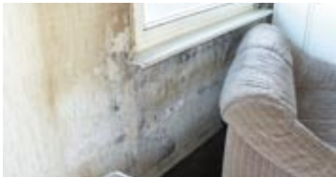
Mould on an external wall behind a sofa
