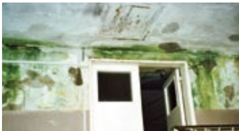
Large areas of mould and algae in a stairwell
